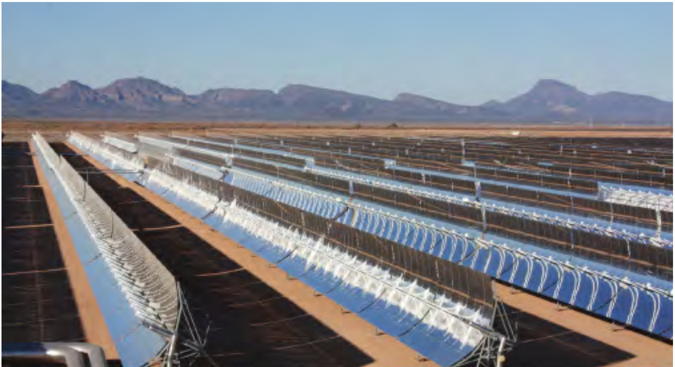
Solana Power Plant west of Gila Bend, Arizona.
